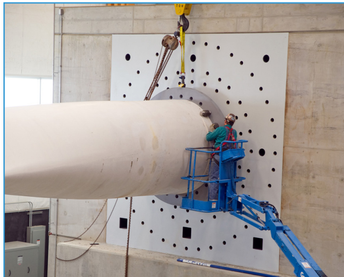
Offshore Wind Laboratory reaction wall
